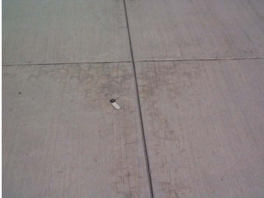
Figure 5. Beginning stages of ASR: early-age cracking at Holloman AFB five years after construction.
