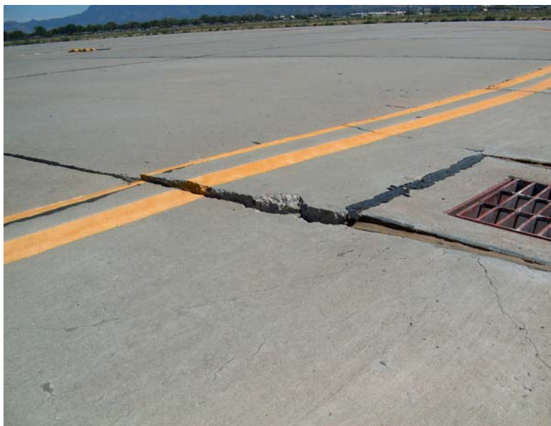
Figure 4. Shoulder heaving from ASR expansion at Seymour-Johnson AFB (top) and damage from ASR swelling pressures at Kirtland AFB (bottom).
