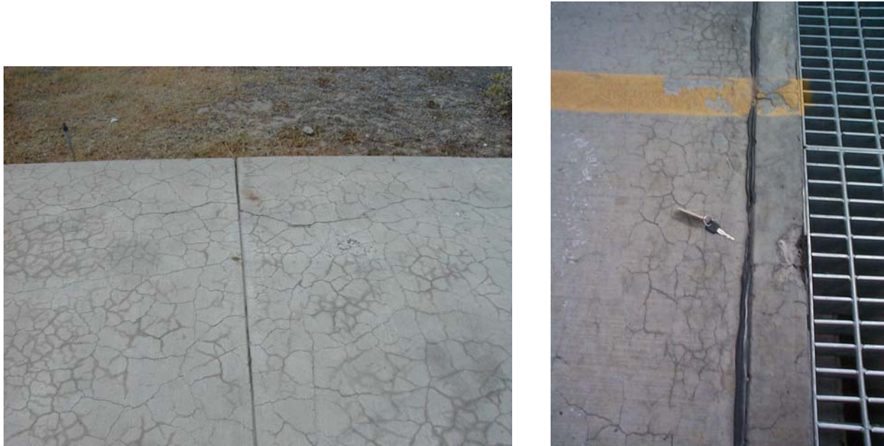
Figure 2. Cracking caused by ASR at Channel Island ANG Station (left) and Holloman AFB (right). Note spalling on the trench drain and the expansion joint squeezed closed on the right by the expansive forces of ASR in the surrounding concrete.
