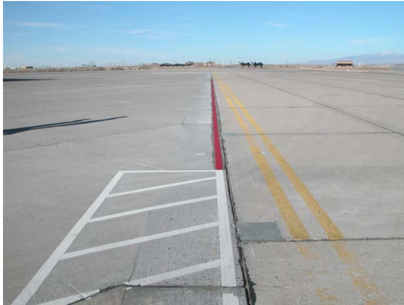
Figure 6. Examples of maintenance for ASR-damaged pavements. Patching (upper left) requires meticulous care to accomplish well, but even with the best technique, patching ASR-damaged pavement is difficult since ASR gel (seen as white deposits in the photograph on the upper left) can inhibit the bond between patch and pavement. Poorly done patches (upper right) soon become a FOD hazard themselves. Heaved areas from ASR swelling can sometimes be ground level (bottom), but such areas are likely to heave again in the future and will require re-grinding.
