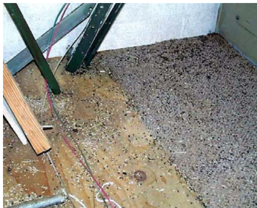
Figure 4. Heavy rodent contamination.
